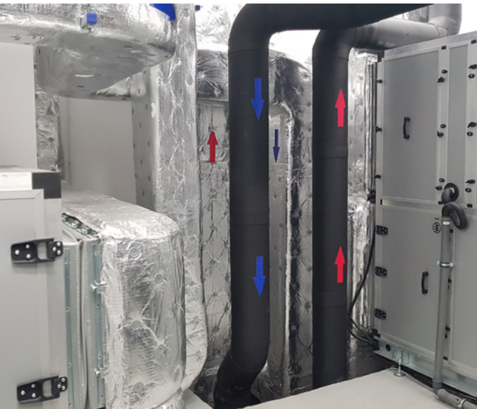
Photograph 2.36. The recuperation system in the Entertainment and Sports Hall in Ryczywół Source: Sławomir Kalinowski.
